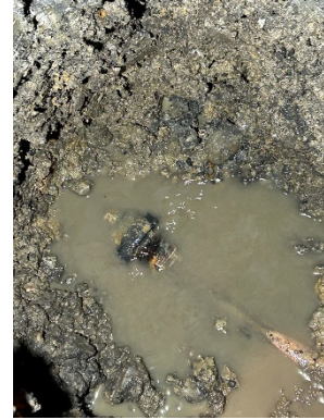
Broken water line at Quantico
